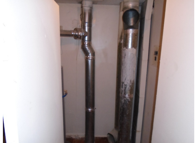
Typical utility closet
